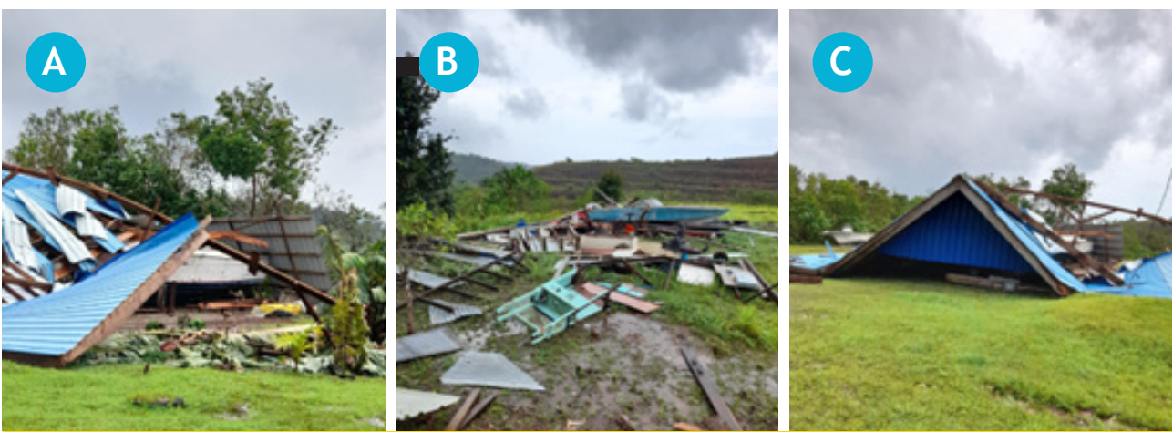
Figure 2: MT Fishing super storm Surigae damage; a) collapsed building; b) building debris; c) collapsed roof; 2021, photos provided by PCOC.
